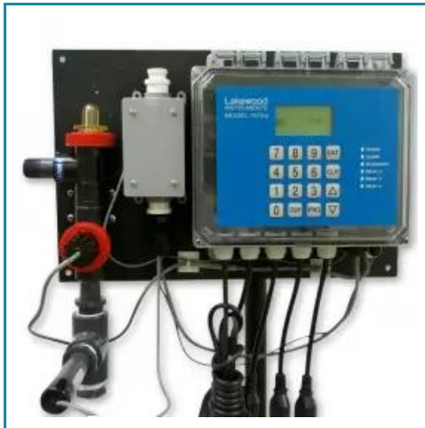
Controller with conductivity sensor and flow switch plumbing assembly on a mounting plate.
